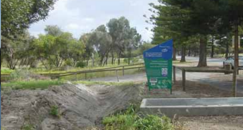
Stormwater outlet, Taperoo
